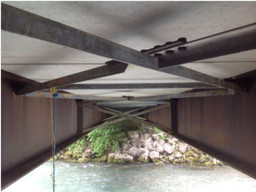
galvanized bracing and diaphragms
