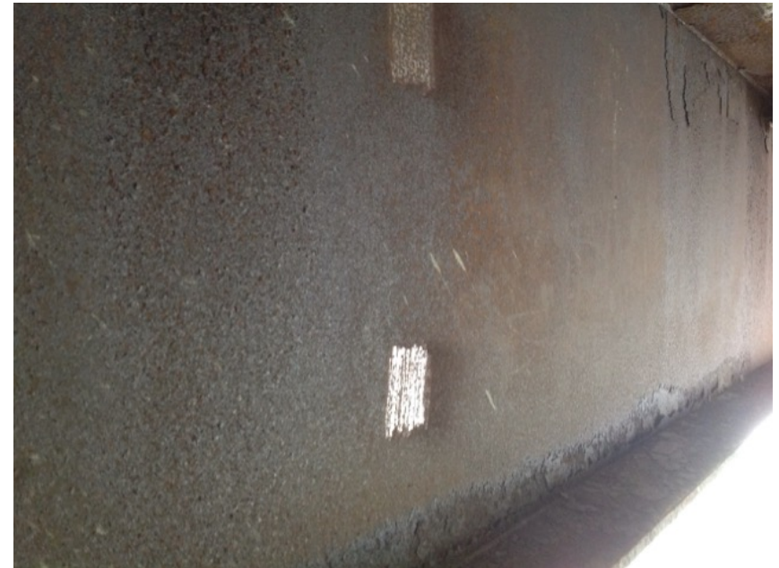
locations of previous web measurements - no further delaminating in these locations
